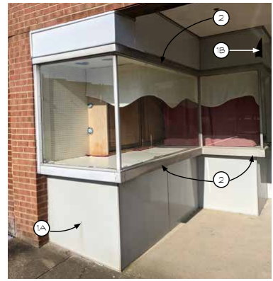
PARTIAL LEFT STOREFRONT Dimensions provided by other. Verify all dimensions in field.
