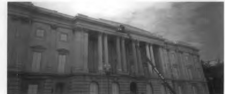
Figure 1. Low-to-medium-pressure steam (hot-pressurized water machinery) is being used in front of the exterior of the U.S. Tariff Commission Building, the first marble building constructed in Washington, D.C., in 1833. This method was selected by an architectural conservator as the "gentlest means possible" to clean the marble. Steam can soften heavy soiling deposits such as those on the cornice and column capitals, and facilitate easy removal. Note how these deposits have been removed from the right side of the cornice which has already been cleaned.
